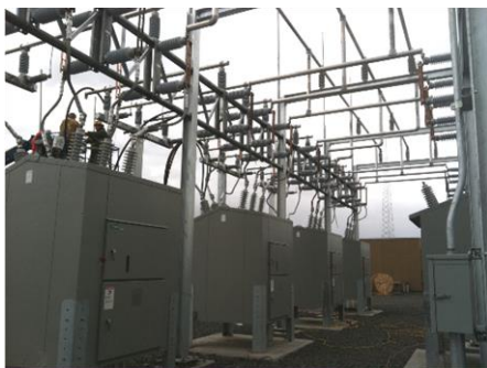
Horse Butte Substation, 2012 Project Manager: Kelly Norman Foreman: Lenny Comstock Picture by Kelly Norman
